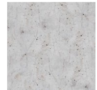
Masonry Concrete Stained
