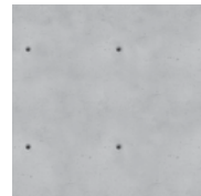
Masonry Concrete Crater
