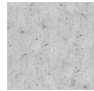
Masonry Concrete Stained
