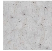
Masonry Concrete Stained
